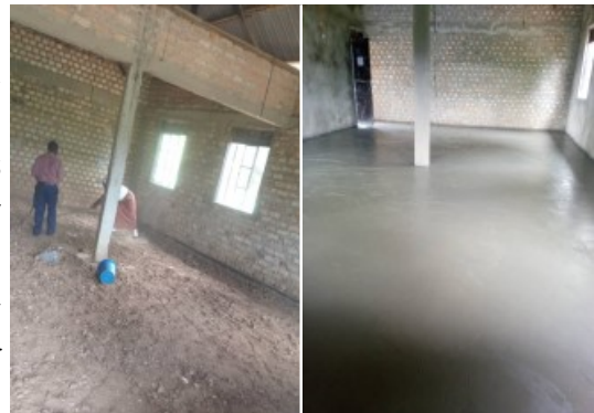
The new classroom: Preparing and levelling the floor and afterwards—ready for students!
